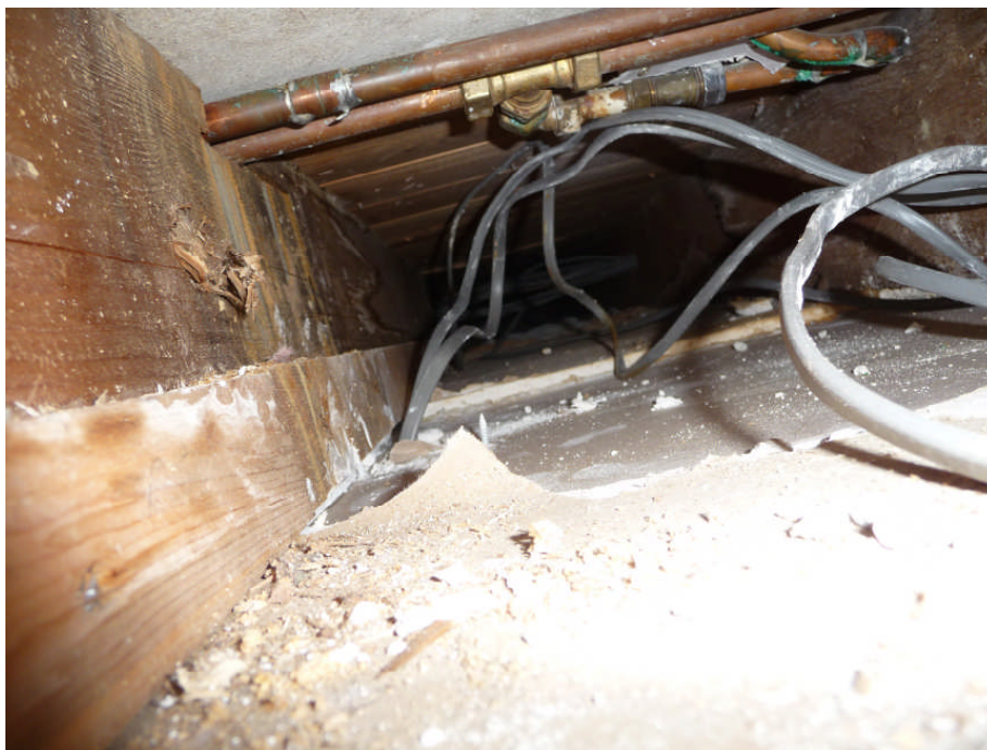
Showing on top of ceiling where leak originated
